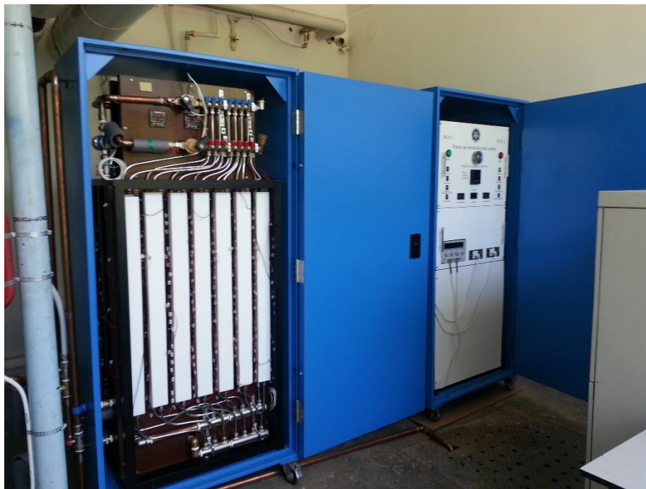
Figure 7. Thermoelectric generators placed in 7 columns
